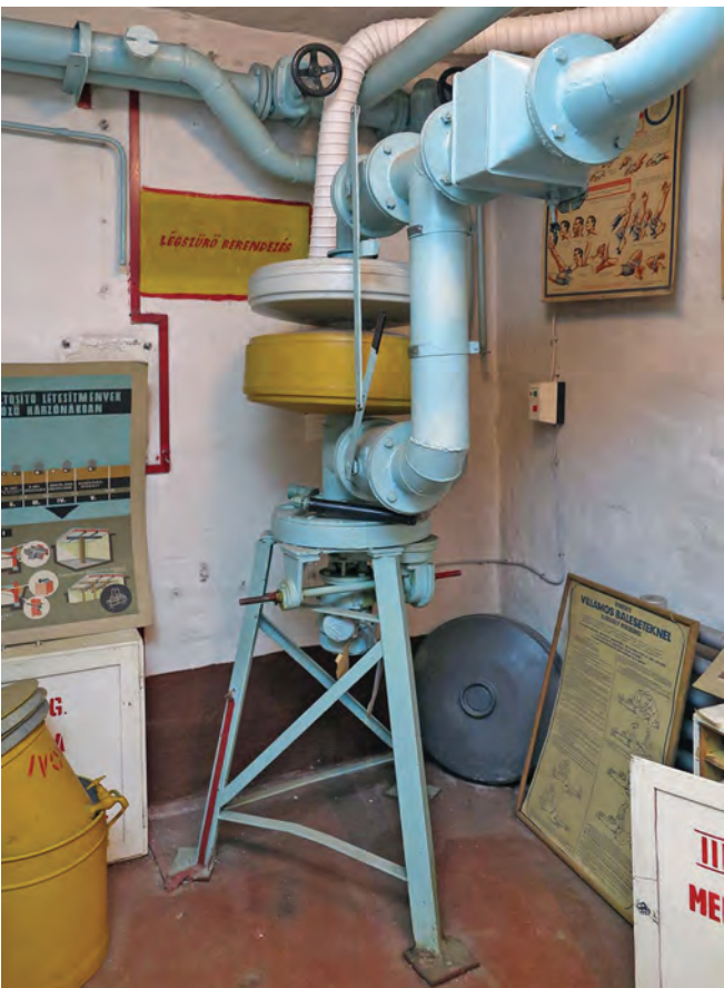
The small scale air-handling plant in shelter number 2 at Csepel with training posters on the walls
